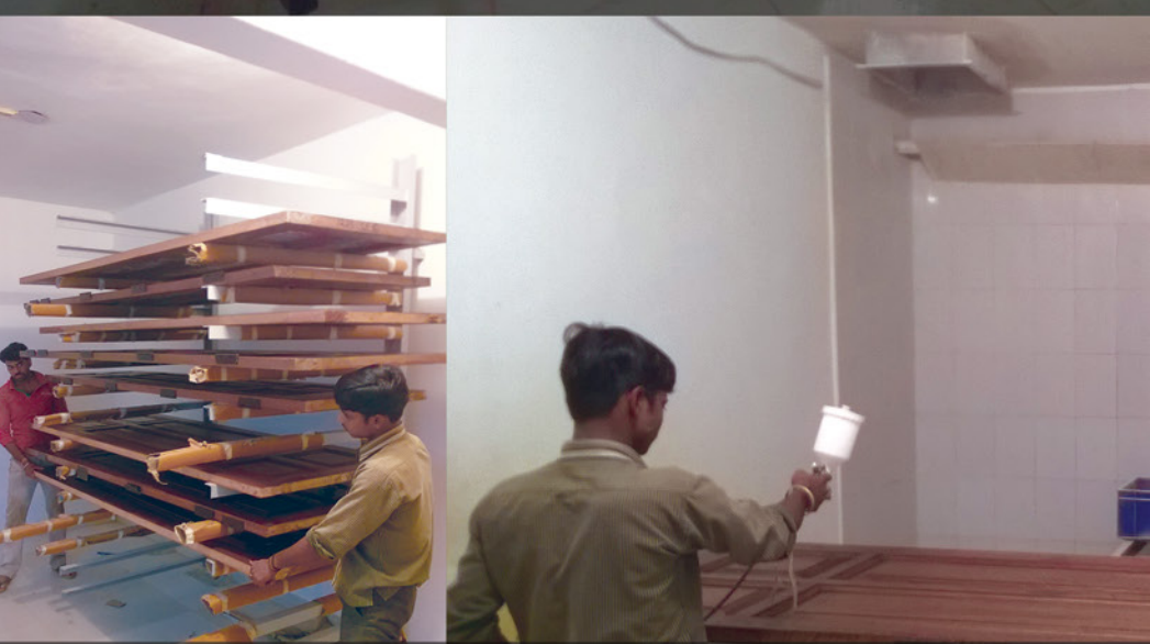
PRESSURIZED POLISH BOOTH A vacuumed, dustless booth in which, paints and polishes are sprayed over doors and windows to give it silky smooth finish.
