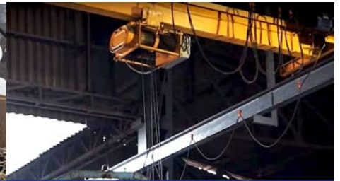
Electric Overhead Crane
